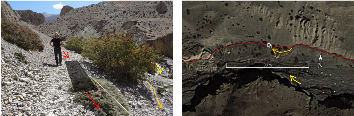
Figure 7.8: Position of the inspection chamber I1 ( x = 210 m; 29^{\circ}05'20.66''N / 84^{\circ}00'38.52''E ). Left: Currently, the open channel runs along a cliff (orange arrow), which is destabilized by water percolating through the soil. The pipeline (red arrows) and the chamber (black rectangle) are proposed to be shifted inwards to be at a safe distance from the instable slope downhill (photo: 27/09/2013, Daniel Bernet). Right: Bird's eye view of the inspection chamber's location. The red line indicates the pipeline, the orange arrow highlights the current routing of the open, earthen channel and the yellow arrow points in Puyung Khola's flow direction (source: Google Earth Pro, accessed 30/01/2014).
