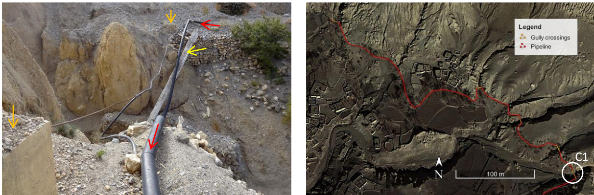
Figure 7.15: Position of the gully crossing C1 ( x = 1649 - 1666 m; 29^{\circ}05'41.25''N / 84^{\circ}00'09.07''E ). Left: The pipeline (red arrow) was fixed on a long wooden bar (yellow arrow), which rested on gabion structures. The base of these gabions was eroded which triggered the crossing's collapse. On the steel rope, held by two concrete anchors (orange arrows), only the drinking pipeline was fixed, which is currently not used anymore (photo: 26/09/2013, Daniel Bernet). Right: Marked location of the gully crossing (source: Google Earth Pro, accessed 31/01/2014).
