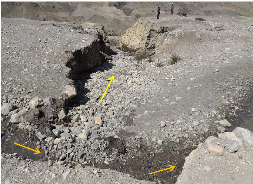
Figure 3.6: Diverting the water from the main channel (orange arrow) into a steep gorge (yellow arrow) draining into the Puyung Khola visibly led to serious backward erosion. This ongoing process has to be stopped immediately, as it is endangering the stability of the current channel and the future pipeline. Therefore, an inspection chamber accommodating a pipeline, safely conveying water back to the Puyung Khola, is proposed (photo: 11/05/2012, Daniel Bernet).
