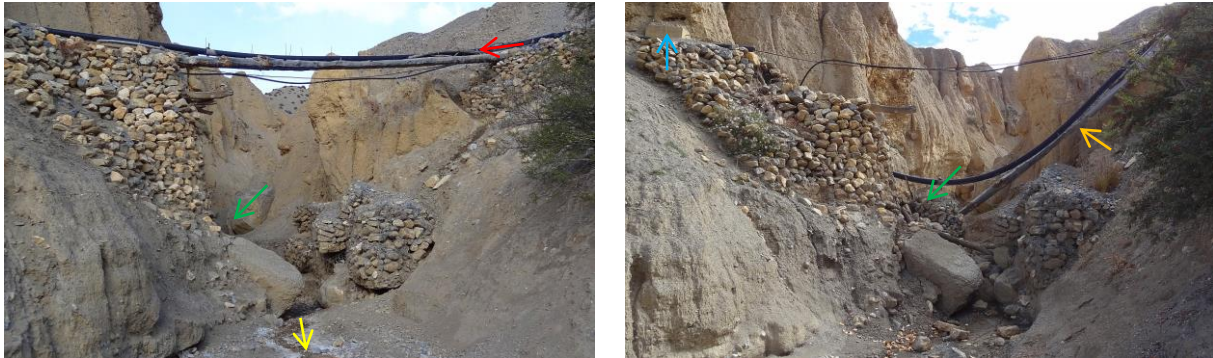
Figure 7.5: Gully crossing (C1) before and after the collapse taken place in summer 2013. Left: The pipeline (red arrow) was fixed on a long wooden bar, which rested on stacked rocks on each side of the gully (photo: 11/05/2012, Daniel Bernet). Right: The base of the structure (green arrow) situated at the gully's right side (relative to the gully's flow direction indicated by the yellow arrow) was eroded, triggering the crossing's collapse. The wooden bar's right end, along with the fixed pipeline, fell into the gully, inactivating the water supply downstream. One of the two anchor blocks, holding the steel rope in place, is indicated by the blue arrow (photo: 27/09/2013, Daniel Bernet).
