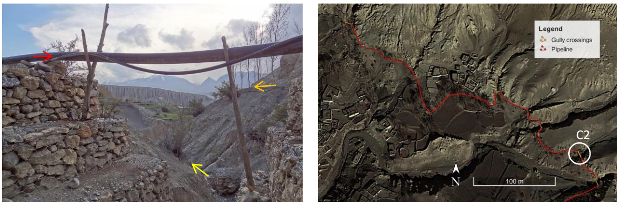
Figure 7.16: Position of the gully crossing C2 ( x = 1685 - 1698 m; 29^{\circ}05'42.26''N / 84^{\circ}00'08.41''E ). Left: The pipeline (red arrow) is supported by two wooden Y-bars standing on stepped gabions on each side of the gully (yellow arrow). The open channel currently in use (orange arrow) can be seen in the background (photo: 11/05/2012, Daniel Bernet). Right: Marked location of the gully crossing (source: Google Earth Pro, accessed 31/01/2014).
