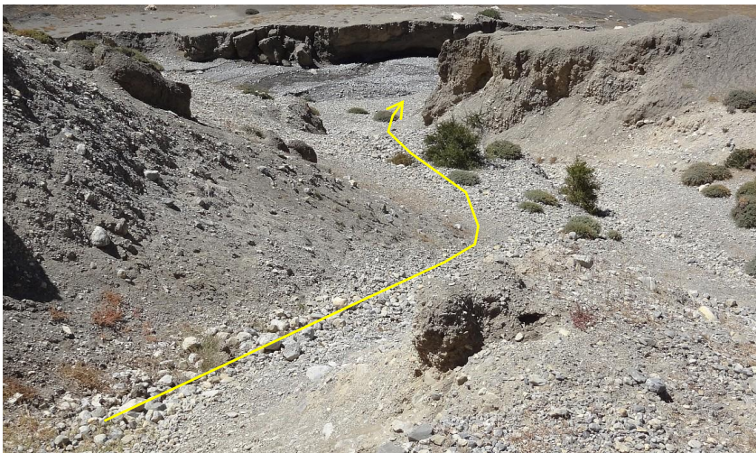
Figure 7.12: The routing of the 95 m long flush pipe connecting the inspection chamber I4 with the Puyung Khola is indicated by the yellow arrow. The installation of this pipe is important, as neglecting the safe discharge might lead to severe backward erosion endangering the stability of the future pipeline (photo: 27/09/2012, Daniel Bernet).
