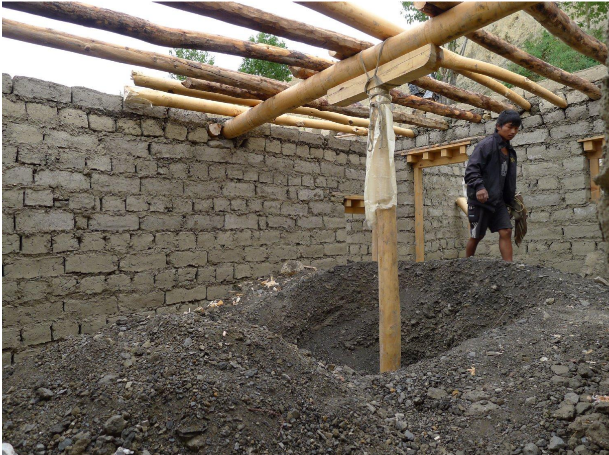
Figure 3.8: Inside view of a house under construction in Yara with earthen walls, wooden poles and part of the wooden slab structure (photo: 03/07/2012, Daniel Pittet).
