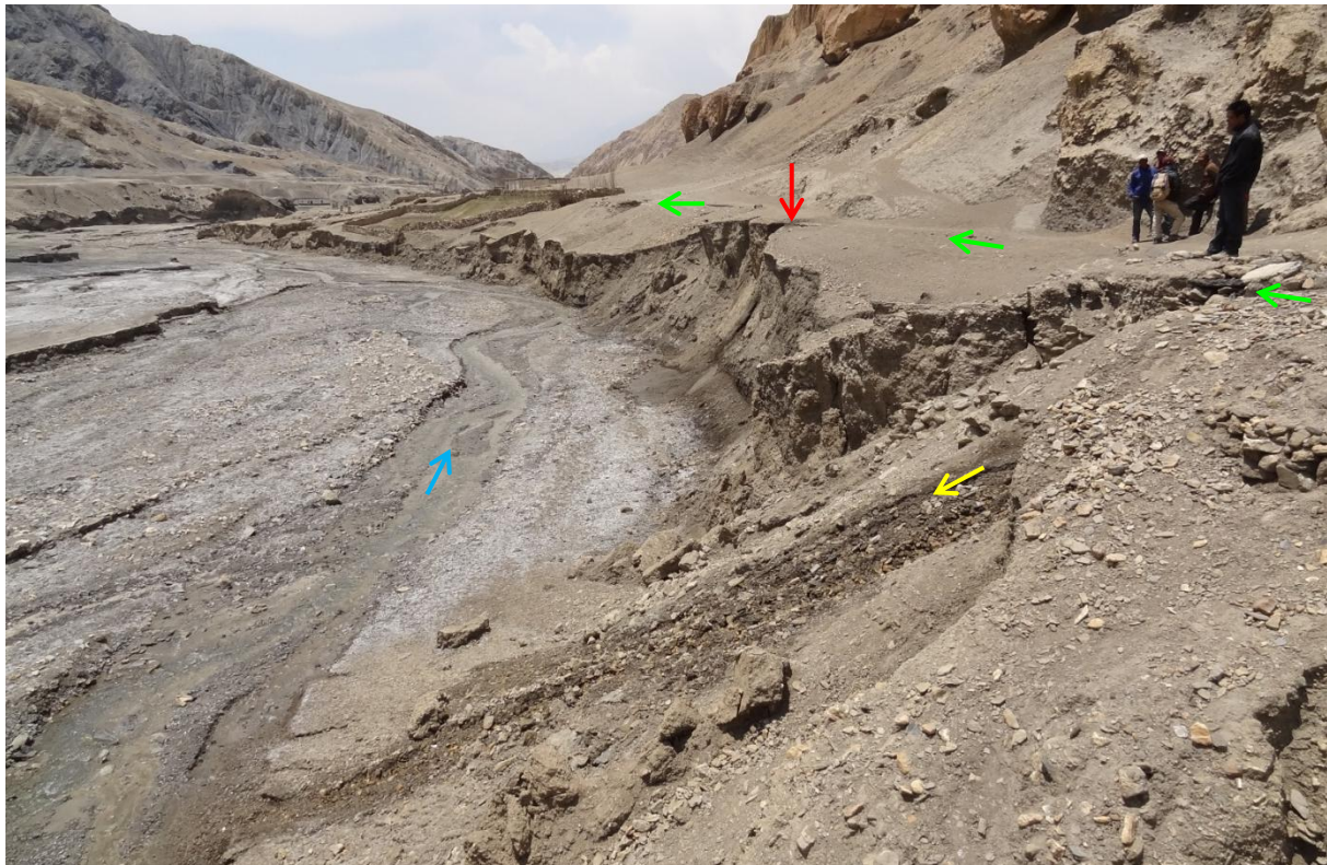
Figure 3.15: View of the piped water distribution line between the reservoir and the village (green arrows, see also section A4 in Figure 3.14 and Table 3.8 respectively) on top of the Samzong Khola's (blue arrow) right riverbank. Particularly the illustrated section (A4) is endangered by different erosion processes. Water draining through gorges uphill is crossing the irrigation system which leads to erosion downhill. Also, numerous leaks in the pipes are washing out soil (yellow arrow) to an extent that the pipes are hanging loosely in the air at several places (red arrow). Finally, during high flow the right river bank is eroded further due to the river's bend decreasing the stability from below. The blue arrow indicates the flow direction of the Samzong Khola (photo: 06/05/2012, Daniel Bernet).
