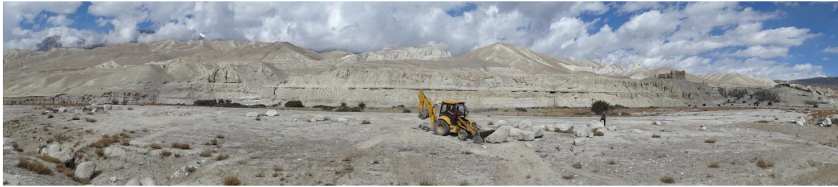
Figure 5.4: Dozer removing large boulders from the agricultural area in Namashung (photo: fall 2012, Tsewang Gurung).
