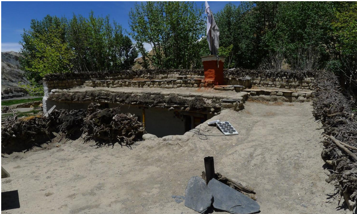
Figure 3.4: Roof top with soil/ash surfacing, wood disposal for drying, solar modules for lighting system, shrine (in red) and pipe for fire smoke evacuation in Samzong. The places corresponding to inside partition walls are covered by flat stones for a better protection against rainwater penetration (photo 28/06/2012, Daniel Pittet).
