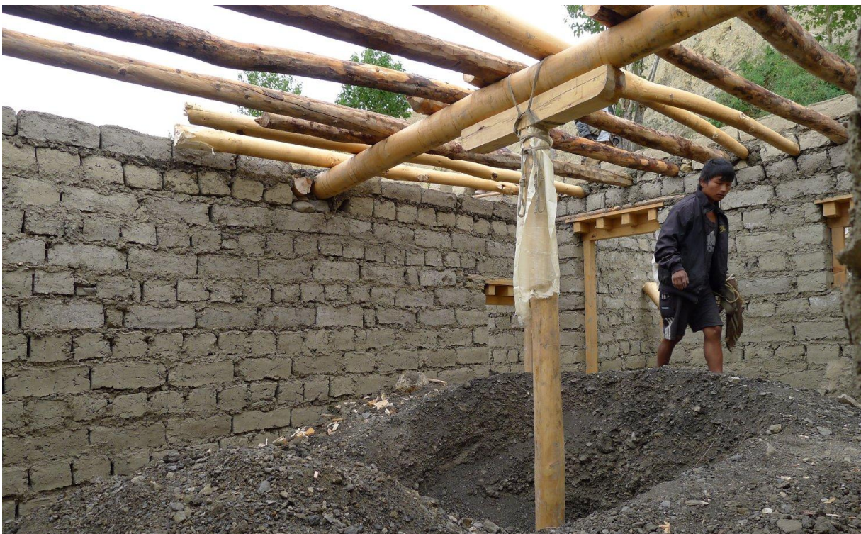
Figure 3.3: Inside view of a house under construction in Yara with earthen walls, wooden poles and part of the wooden slab structure (photo: 03/07/2012, Daniel Pittet).
